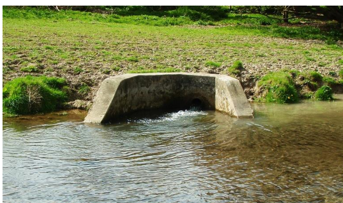
STW Outflow – upstream of Site 3
